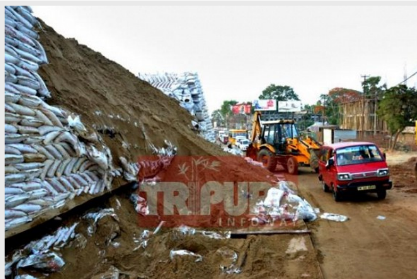
PHOTO : Nagarjuna Construction's Load testing failed on Thursday at Bordowali, Agartala TIWN Pic April 21
