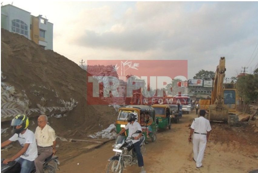
Sandbags colloapsed, Load testing failed at Bordowali on Thursday. TIWN Pic April 21
