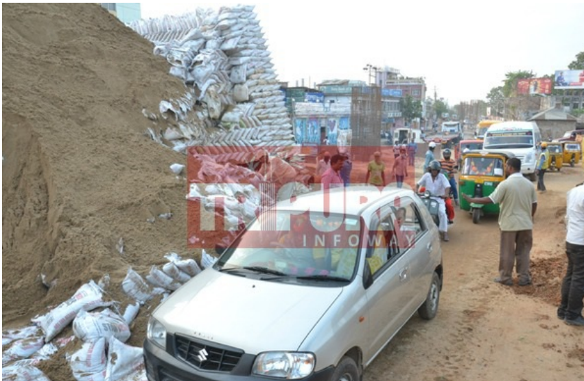
Sandbags colloapsed, Load testing failed at Bordowali on Thursday. TIWN Pic April 21
